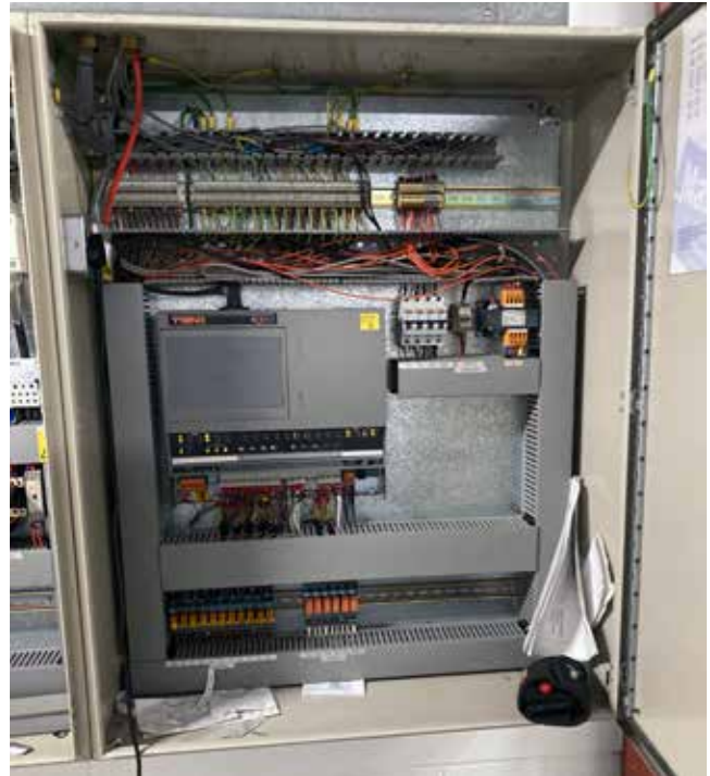
Figure 2 - one of the BMS panels upgrade. The panel itself was in good condition so many components were reused to deliver the customer good value for money
